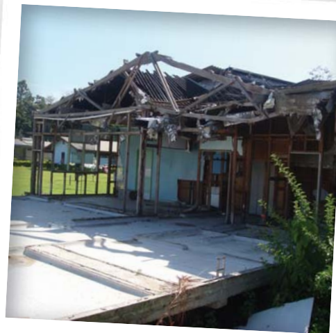
Fig. 1. Photograph of ward at Lae Hospital, Lae, which is under-resourced and in need of repair.
